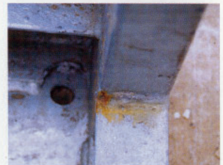
Fig 4: Seepage from pretreatment solutions from a weld
