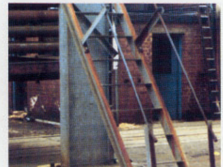
Fig 5: Water draining from rusting steel (out of picture) causes staining of sound galvanized surfaces of the stairway illustrated here.
