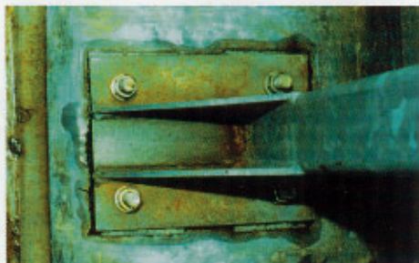
Fig 2b: This staining is superficial and can be removed to expose a sound galvanized coating beneath.
